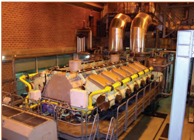
The converted 51/60DF engine at the TMG SPE cogen plant. The newly installed gas supply lines are clearly visible in their mandatory yellow color coding.
