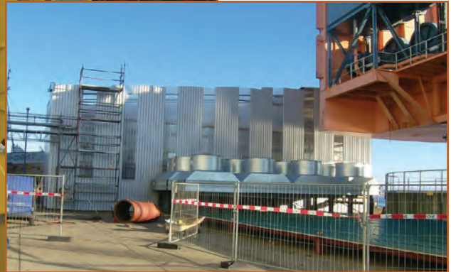
One of the two facilities used to house the Caterpillar 16CM32 engines at the Rostok test site in Kiel, Germany.
