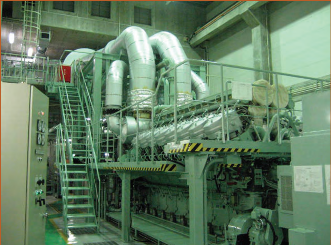
Two Niigata 16V32CLX diesel engines are operating at the two power plants of Kyushu Electric Co. Ltd.
