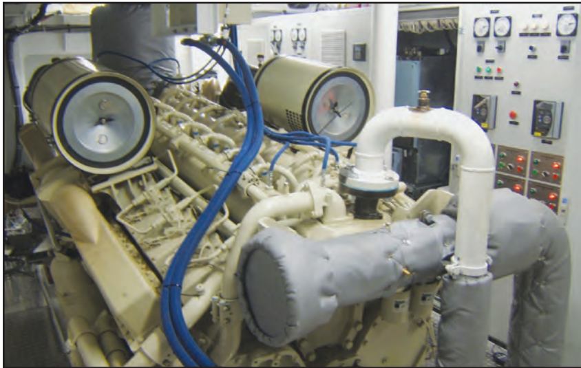
A view of one of the two Cummins QSK50 main diesel engines; each produces 1342 kW at 1800 r/min. In this hybrid system, these engines are used to power mechanical drive propulsion system as well as recharge the batteries. In the background is the housing for the power management system, which fills the center of the engine room.
